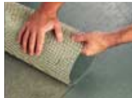
Step 1: Unroll the Everlay on the concrete, laying the rolls alongside each other.
